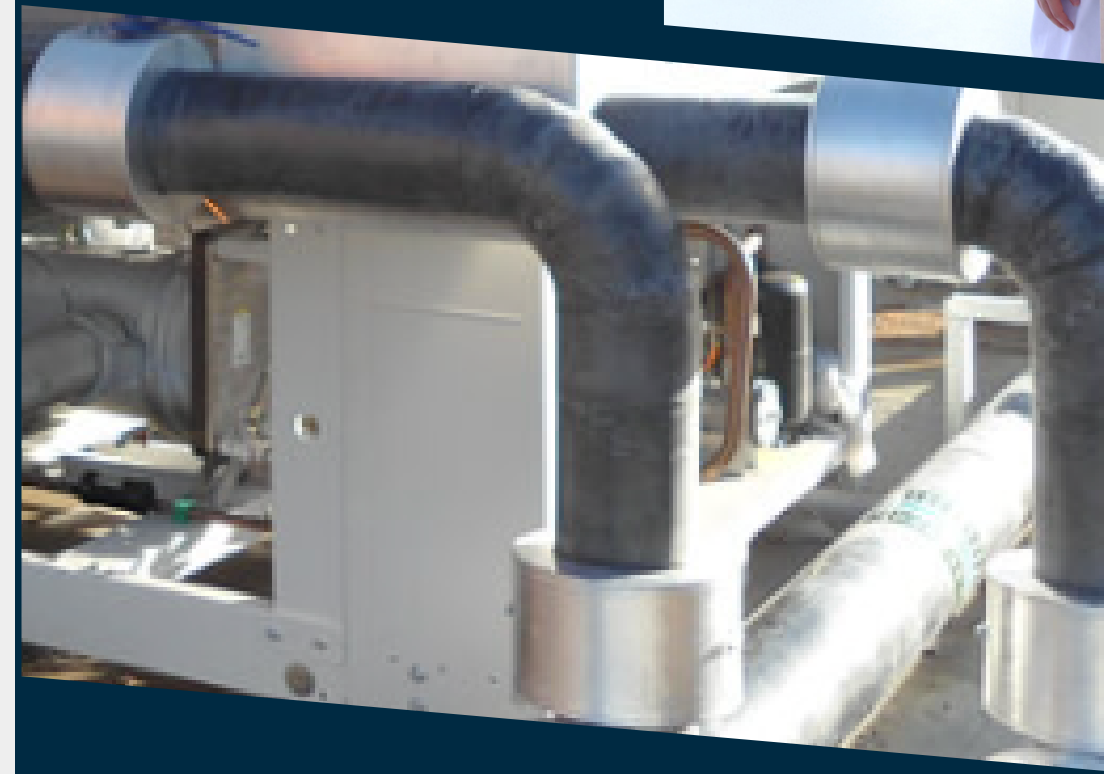
Centralized Cooling System
